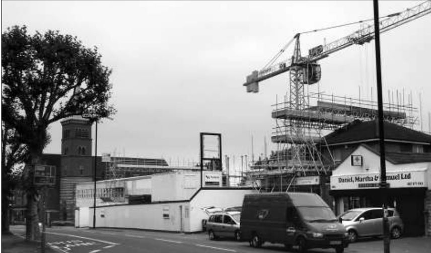
Local photographer Allan Keen is capturing the development of the former Texaco garage site on the Wells Road. In his second picture the scaffolding for the flats and retail development is rising above the Wells Road. Photograph by Allan Keen (allankeen@blueyonder.co.uk)
